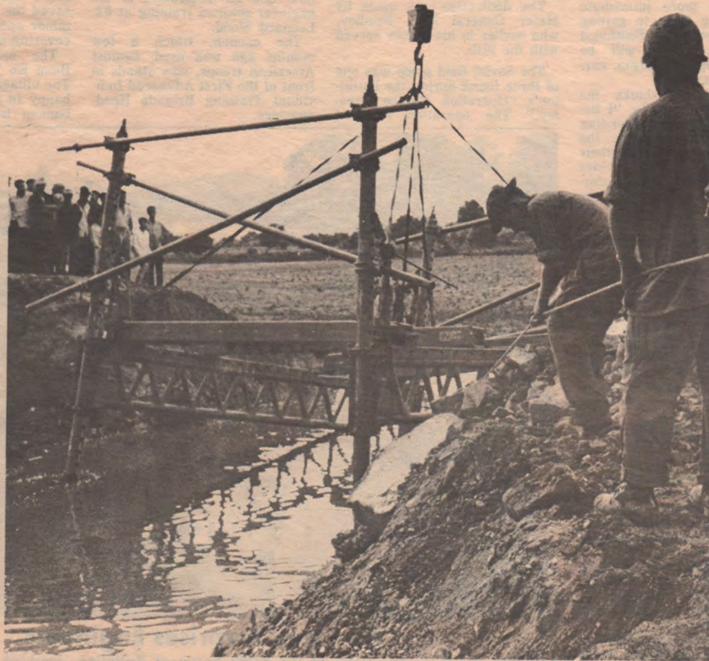
FINISHING TOUCHES —With the bridge firmly implanted, engineers prepare to add the last touches to the temporary passageway.
