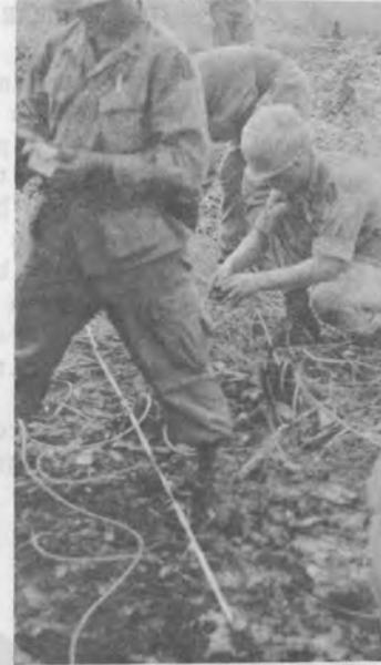
After charges are in place, detonating wires are secured to insure proper size of the blasting pattern is achieved.
