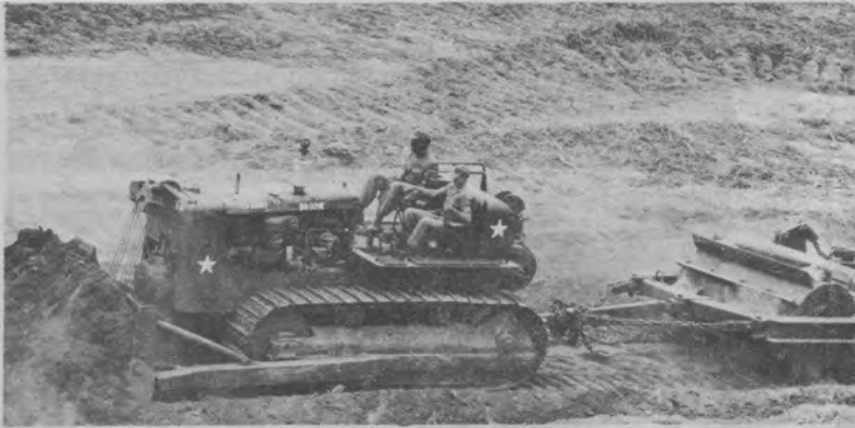
EXPERIENCE IS WHAT COUNTS – Clearing infantry training area requires heavy equipment and experienced operators.
