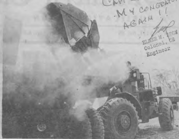
DUST AND DIRT — An earthmoving operation of the 518th is not a job for one who is afraid of a little dust and dirt.
