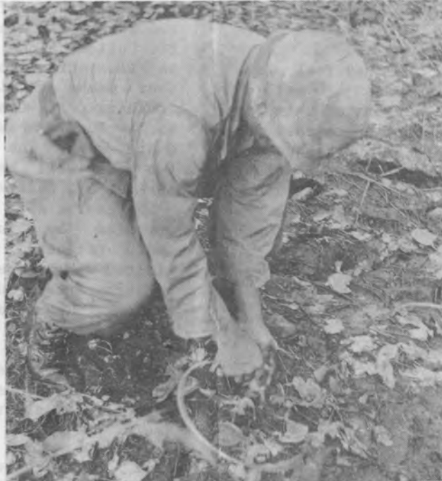
Charges are implanted after spacing and loading techniques are carefully examined. A "stacking" technique was also tried.
