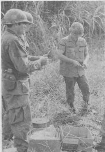
While boreholes were being prepared, these Engineers ready detonators to be inserted. Holes were carefully punched in charges so detonating wires could be fixed.
